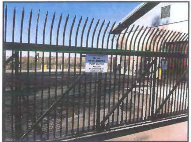
View of City of West Sacramento Water Booster Pump Station on APN 067-180-024
